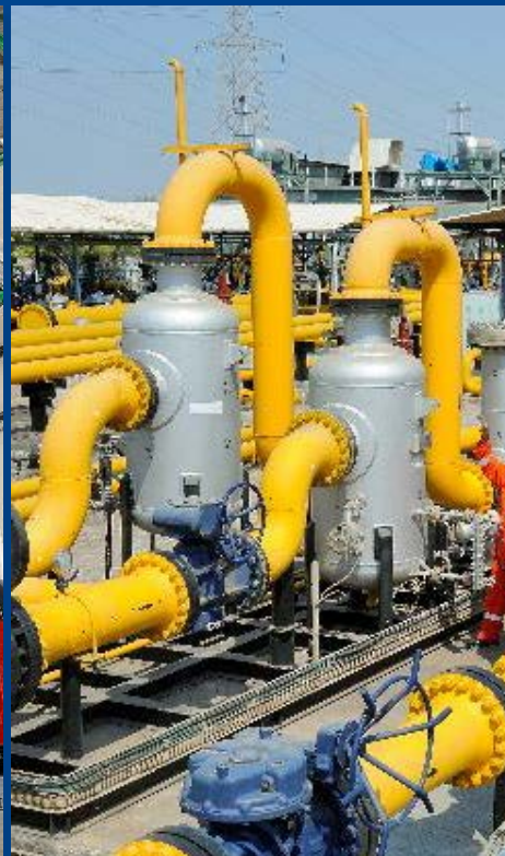
Natural Gas Skid
